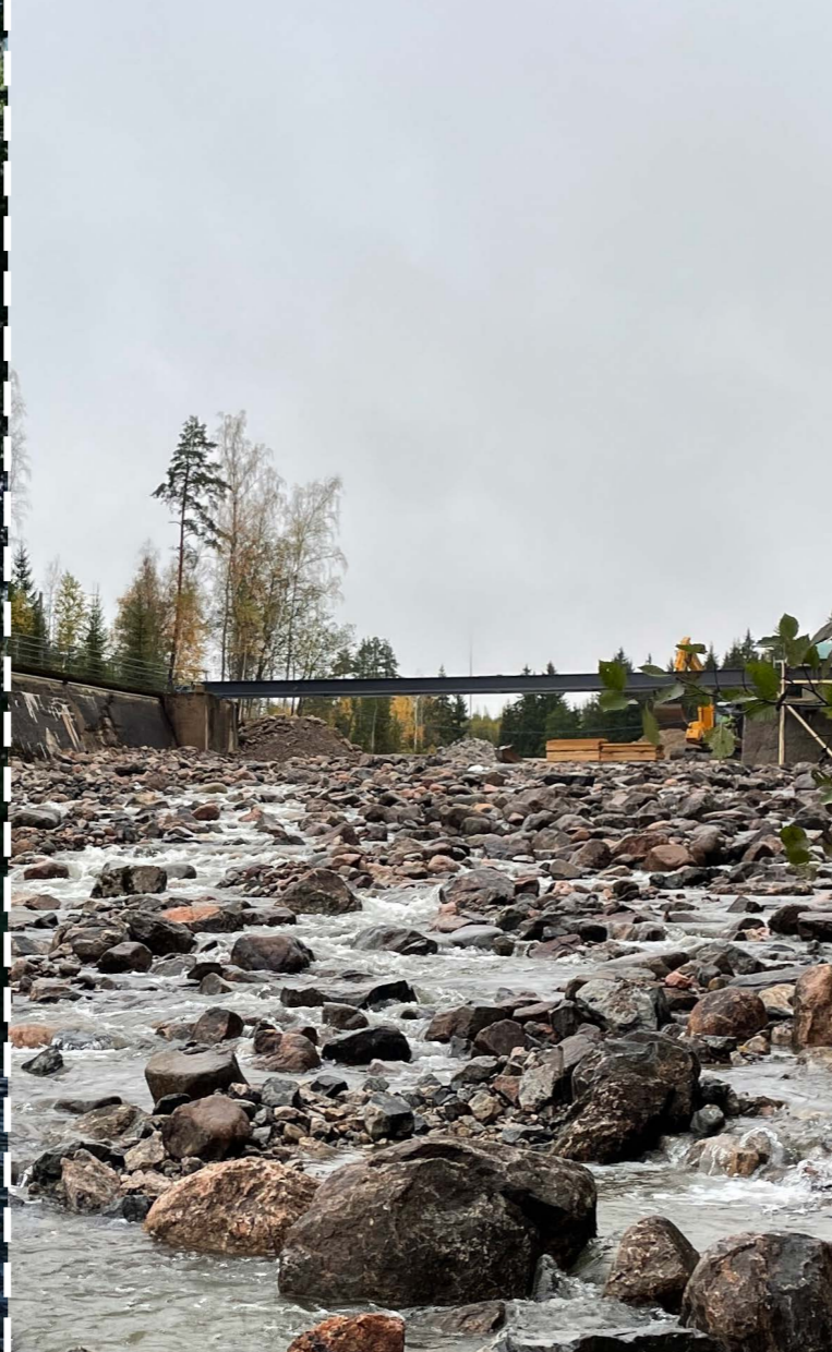
The removal site at Hiitolanjoki River, Finland: (left) before and (right) after the removal operations of the Lahnasenkoski Dam in August 2022 © Hanna Ollikainen
